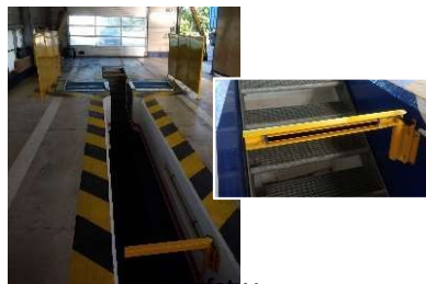
Pit safety : Infrared barrier Mounted on swing gate
