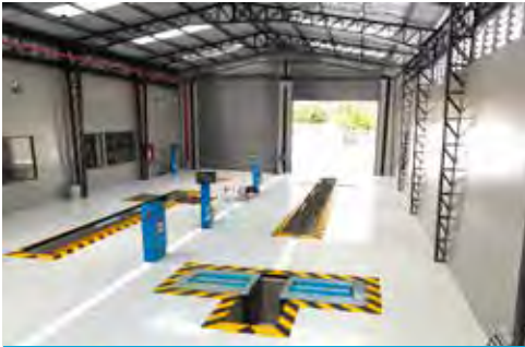
LV | HGV FULL TEST LANE
